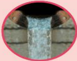
Aggravation of natural disasters (drainage system blockages)
